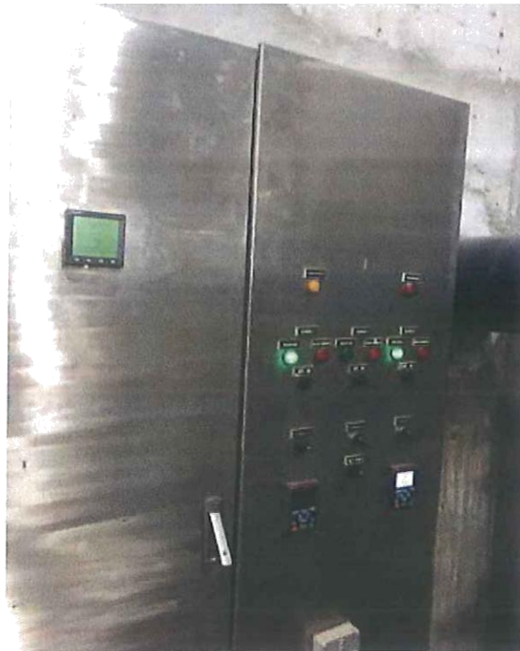
Figure 11.-Tablero de control Reservorio EB Norte
