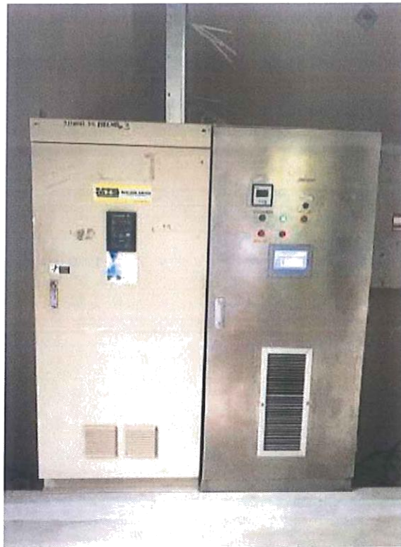
Figure 6.-Tablero de control EB Banco de Arena #3
