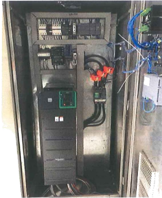
Figure 7.-Elementos de tablero de control EB Banco de Arena #3
