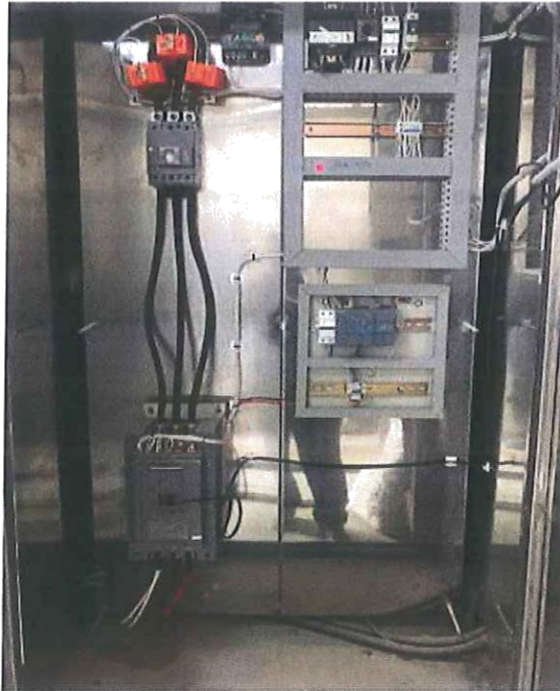
Figure 9.- Elementos de tablero de control EB Norte
