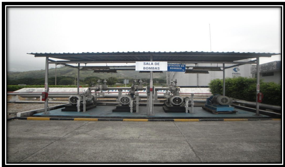
Figura 5: Sala de Bombas en Terminal Fuel Oil.
